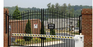
Gate Monitoring & Control
