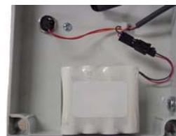
Figure 8-6 – WPR Battery Pack Connected
